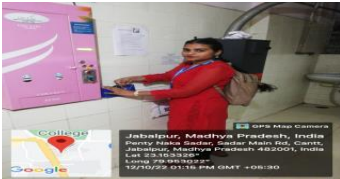
Plate 3: Sanitary vending machine in the premises
